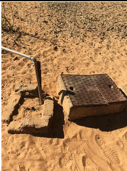
Figure 9.27 Piped Water in the Project Area
