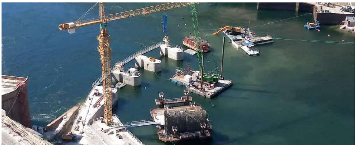
KDRP - Progress on the Cofferdam construction works with Pier 2, Pier 3 and Pier 4 all complete
