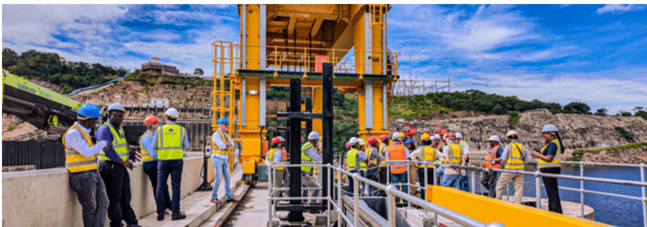
KDRP site visit undertaken by participants of the Joint Mission, comprising technical experts, financiers and engineering teams, to assess progress regarding the Kariba Dam Rehabilitation Project spillway refurbishment works.
